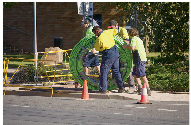
Fig. 1. Workers bury new fiber optic cable in Wagga Wagga, NSW, Australia. The high cost of installing such cable has helped drive research into expanding the amount of information existing optical fiber networks can carry. Credit: Bidgee, Wikimedia Commons (CC BY-SA 3.0 AU).
