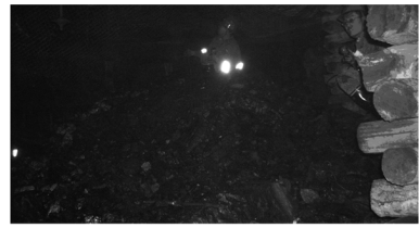
图7 保德煤矿88303回风巷冒顶实例 Fig. 7 The roof falling of 88303 return air roadway in Baode Colliery
