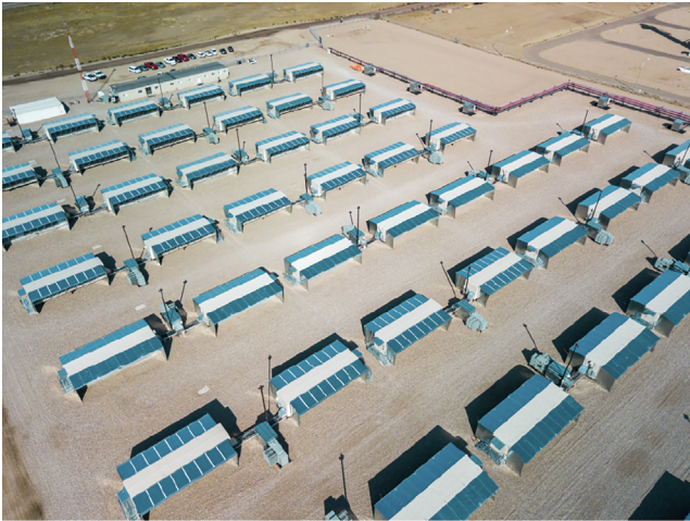
Fig. 1. This Bitcoin mining facility—Canada's largest—covers about 4.5 ha in Medicine Hat, AB. Drawing more than 63 MW at any given time, the operation consumes roughly the same amount of electricity as the town of Medicine Hat with its population of 63 000. Credit: Wikimedia (CC BY 4.0).
