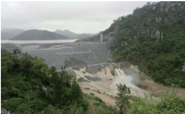
Fig. 8. The failure of the Tokwe Mukosi Dam.
