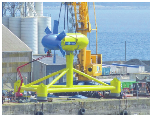
Fig. 6. Sabella D10 tidal turbine dockside in Brest, before installation (photo courtesy of Erwann Nicolas (Sabella, France)).
