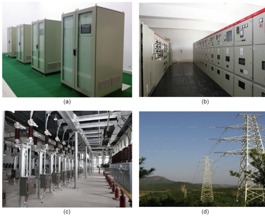
Fig. 2. Equipment and facilities of the WEM transmitting station. (a) The 2 \times 500 kW transmitter; (b) the control cabinet; (c) the antenna tuning room; (d) the feeder tower.
