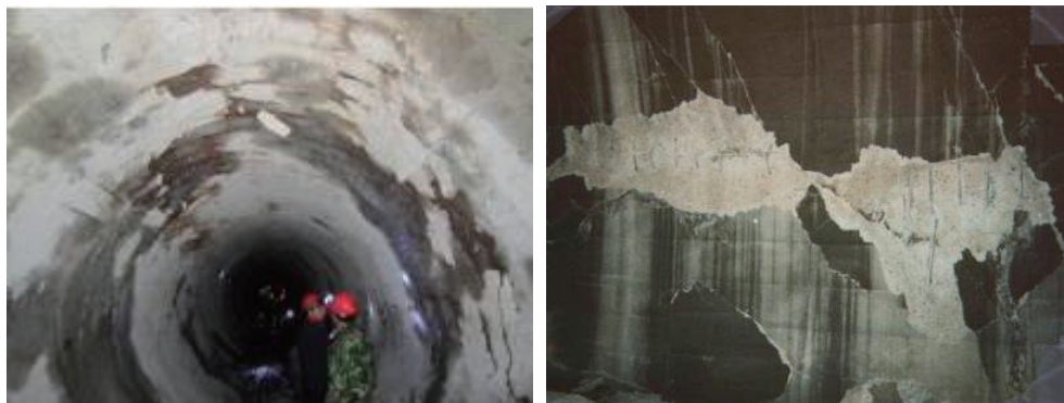
(a) Carbonation of concrete and corrosion of reinforcement
