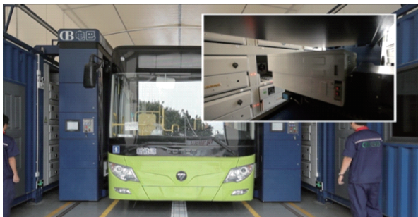
Fig. 8. Containerized battery charging/swapping station.
