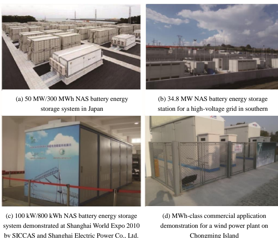
Fig. 1. Commercial application of NAS battery energy storage system/power station.
