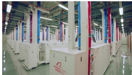
Fig. 8. Alibaba Cloud immersion liquid cooling server.
