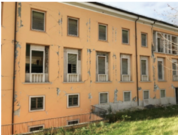
Fig. 12. A damaged building that did not collapse but remained unused after the Amatrice earthquake of 2016.
