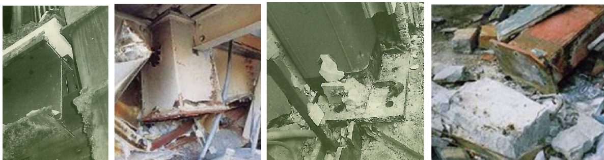
Fig. 7. Failure of steel structures in the Great Hanshin earthquake [7].
