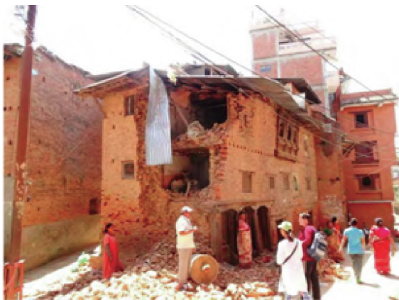
Fig. 1. Unreinforced masonry building damaged in the Gorkha earthquake in 2015 [3].
