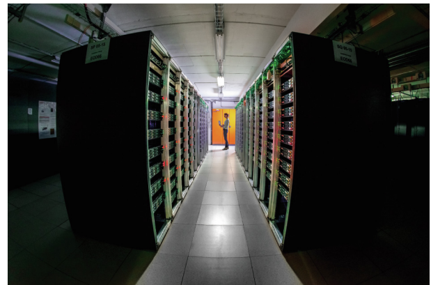
Fig. 1. A look inside the data center serving the vast particle physics laboratory European Organization for Nuclear Research (known as CERN) near Geneva, Switzerland. To handle skyrocketing traffic to, from, and within such data centers worldwide, the photonics industry currently plans to double or quadruple data capacities of laser-based transceivers about every two years. Credit: ©Robert Hradil and Monika Majer/ProStudio22.ch, CERN, with permission.
