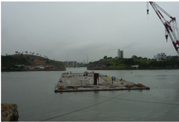
Fig. 2. Transportation of an immersed tube by controlling the hauling cable of the winch at the river bank.
