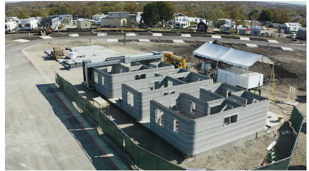
Fig. 3. Icon’s Vulcan II 3D printer, at the far end of the three structures, was used to create the walls of three 37 m 2 homes with different floor plans on a single foundation in Austin, TX, USA. Credit: Icon, with permission.
