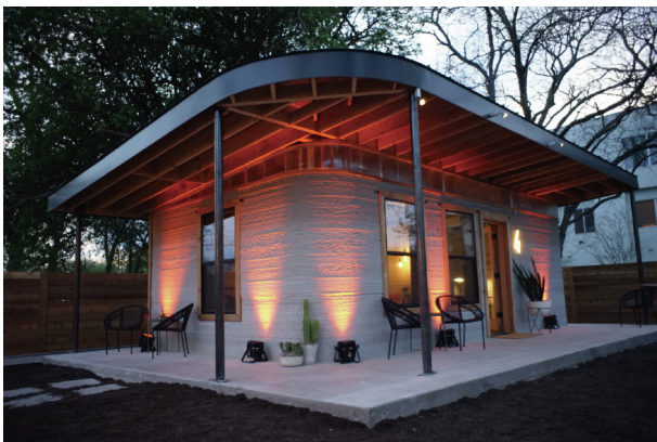
Fig. 2. The Icon (Austin, TX, USA) Vulcan II 3D printer deposits a 2.5 cm × 5 cm line of a concrete-based material called “lavacrete” to build the walls of 37 m 2 houses, like this completed one, in about 24 h. Credit: Icon (press release).
