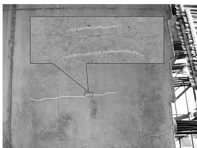
图12 腹板水化热裂缝 Fig.12 Hydration heat caused crack in web
