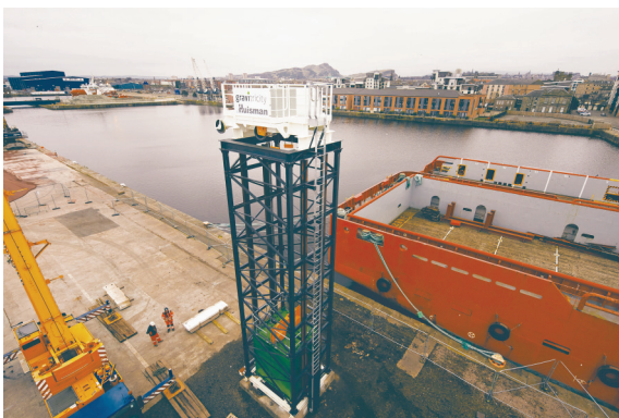
Fig. 2. Gravitricity’s grid-connected, 250 kW GES demonstrator uses two 25-tonne masses suspended within a 15 m tower. Credit: Gravitricity, with permission.
