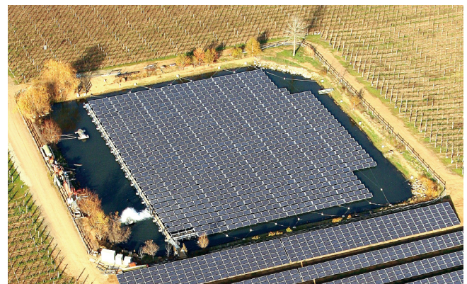
Fig. 2. This small-scale floatovoltaic system covers a pond at the Far Niente Winery in Napa Valley, CA, USA. Containing nearly 1000 panels, the array and the land-based panels next to it produce up to 400 kW of power, enough to meet the winery's electricity needs. Credit: SPG Solar (CC BY-SA 3.0).
