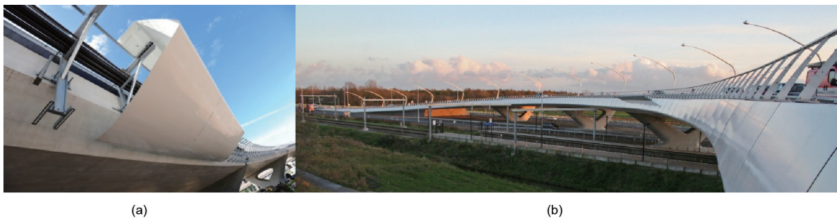
Fig. 8. (a) Installation and (b) final assembly of the edge elements in the fly-over Waarderpolder.
