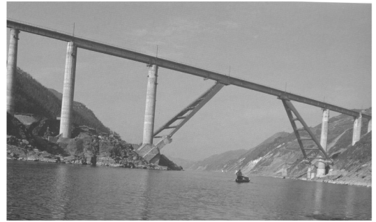
图 7 汉江斜腿刚构铁路桥 Fig.7 Rigid frame with inclined legs railway bridge at Hanjiang
