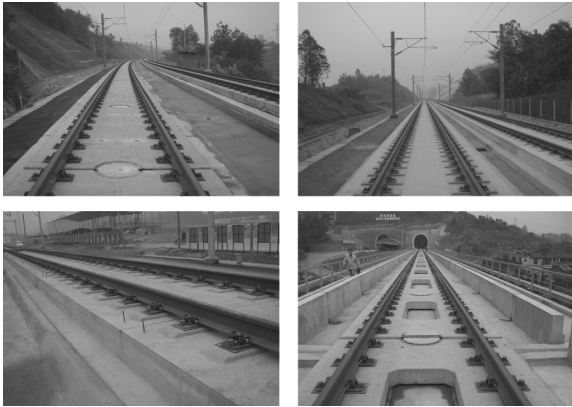
图 46 遂渝线试验段铺设的无砟轨道 Fig. 46 Ballastless tracks laid on experiment section of suiyu line
