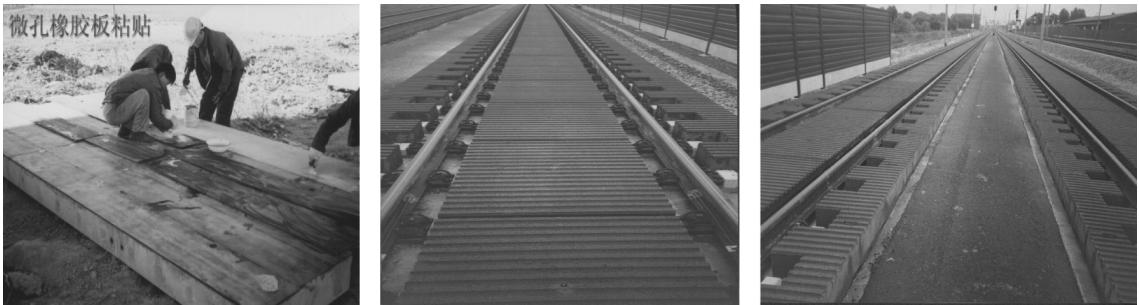
图 17 无砟轨道线路的降噪措施 Fig. 17 Noise reduction measures along ballastless tracks
