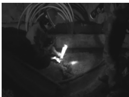
图 17 隧底注浆孔吹风 Fig. 17 Strong wind from tunnel bottom
