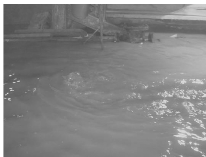
图 18 溶洞段隧底钻孔冒水 Fig. 18 Confined water from tunnel bottom
