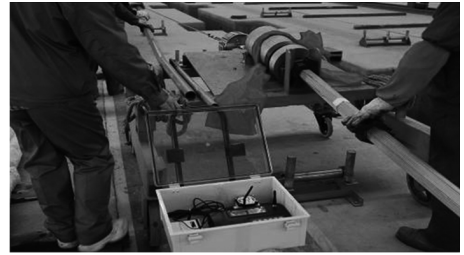
图 9 测力装置和无线发送装置 Fig. 9 Stress detection sensor and wireless transmitter for super-long and super-strong cable
