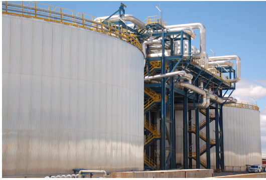
Fig. 3. Two-tank molten salt TES system of Andasol 3 50 MW CSP plant in Spain. Storage capacity: ~28 500 metric tons Solar Salt for 7.5 h storage. Source: Andasol 3.
