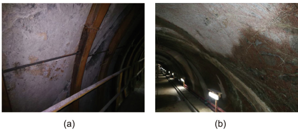
Fig. 12. Macro characteristics of the rock in the 142 + 860–142 + 920 range of the tunnel. (a) Surrounding rock at 142 + 862 and (b) surrounding rock at 142 + 910.
