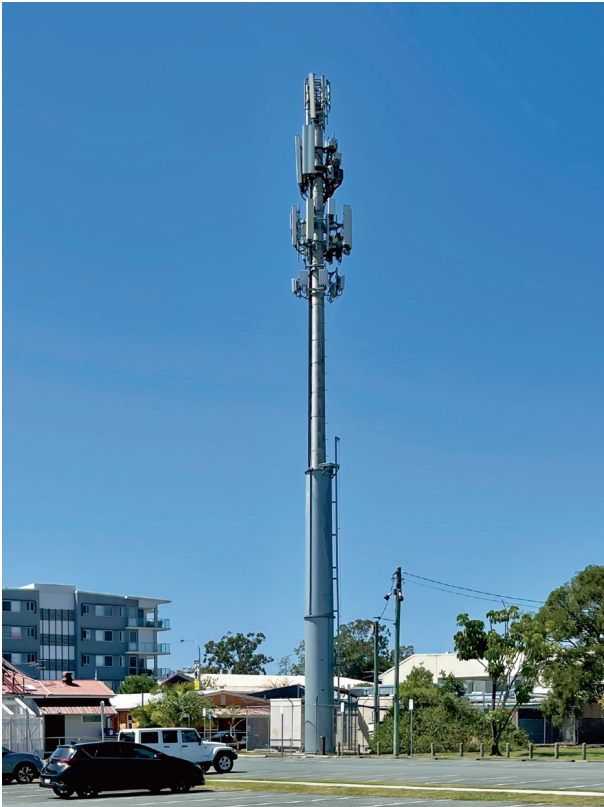
Fig. 2. This 5G base station in Australia receives signals from users' cell phones and passes them on to the network core so they can be routed to their destinations. Some 5G frequencies require large numbers of base stations in a small area because of interference from buildings and other objects in the environment. Credit: Kgbo/Wikimedia Commons (CC BY-SA 4.0).
