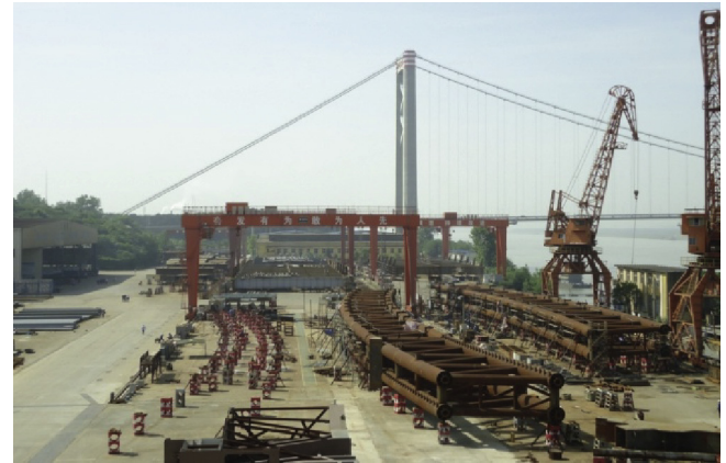
Fig. 9. Coupling fabrication for the horizontal assembly of the lifting segments of the arch truss.
