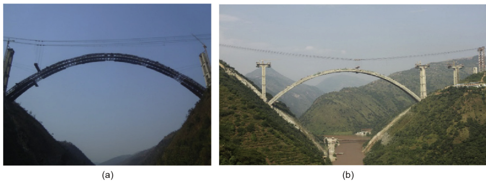
Fig. 15. The (a) stiff skeleton and (b) concrete arch ring of the Yunnan–Guangxi Railway Nanpan River Bridge.
