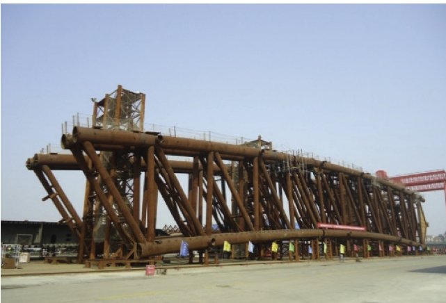
Fig. 8. Coupling verification for the vertical assembly of the lifting segments of the arch truss.
