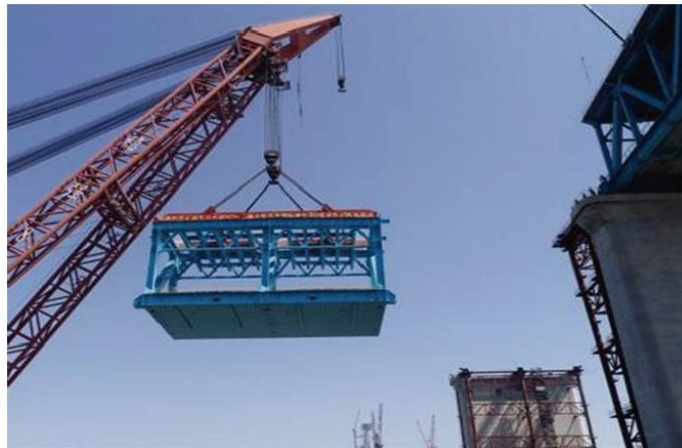
Fig. 4. Assembly and integral hoisting of steel beam segment of dual-purpose highway–railway bridge.
