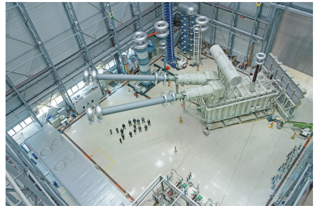
Fig. 2. This is one of the two giant transformers for the new 1100 kV transmission line that runs 3293 km between Xinjiang and Anhui in China. Located at the terminus of the line, it is 37.5 m long and weighs more than 816 t. With > 99% efficiency, the transformer converts the ultra-high-voltage line’s direct current into AC that is distributed to cities. Credit: Siemens (press release).
