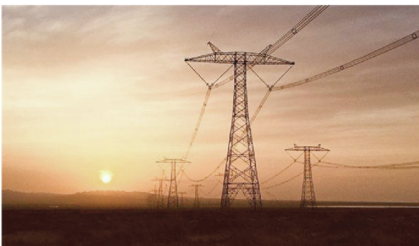
Fig. 1. China has aggressively expanded its high-voltage transmission capacity in the past two decades. Seen here is part of the newly operational ultra-HVDC 1100 kV transmission line. It is the longest, highest voltage line in the world, linking Xinjiang in the northwest part of China to Anhui in the eastern part of China, spanning a distance of 3293 km. Credit: People’s Network–Hubei Channel, 28 September 2019.
