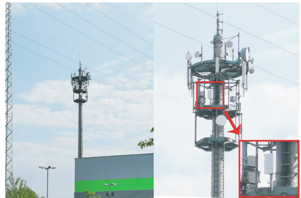
Fig. 3. The transition to 5G networks has started; as of February 2020, cities in at least 34 countries have deployed some 5G [4], including this August 2019 5G upgrade (3.5 GHz, Band n78) on a cell tower in Karlsruhe, Germany. Credit: Tomas Freres, Wikimedia Commons (CC BY-SA 4.0).
