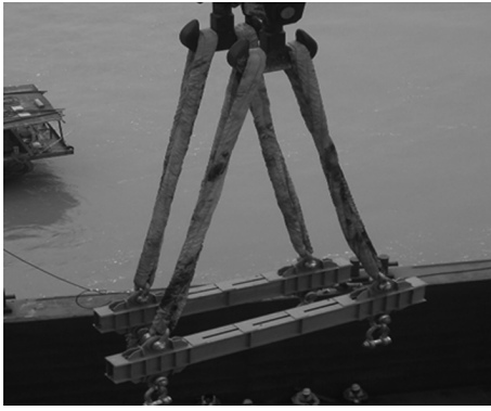
图4 吊带、吊具联接示意图 Fig. 4 Connections of the lifting belts and hangers
