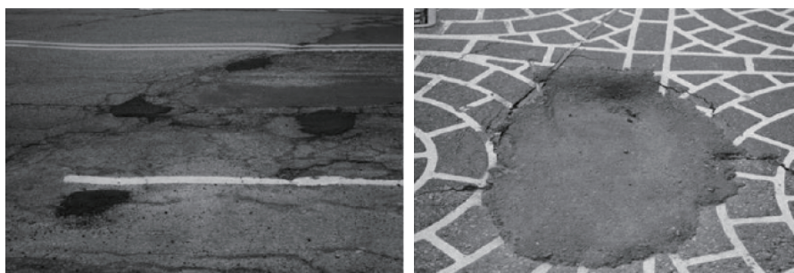
(a) 坑槽的反复修补
