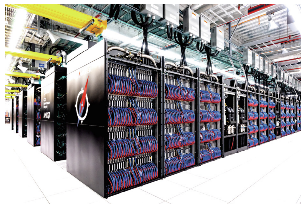
Fig. 1. A view from outside of Frontier shows several of the 74 Cray cabinets, each weighing more than 3600 kg, that make up the supercomputer. The machine features 2.0 GHz central processing units (CPUs) and 1.7 GHz graphics processing units (GPUs), all made by Advanced Micro Devices. Credit: Oak Ridge National Laboratory (CC BY 2.0).
