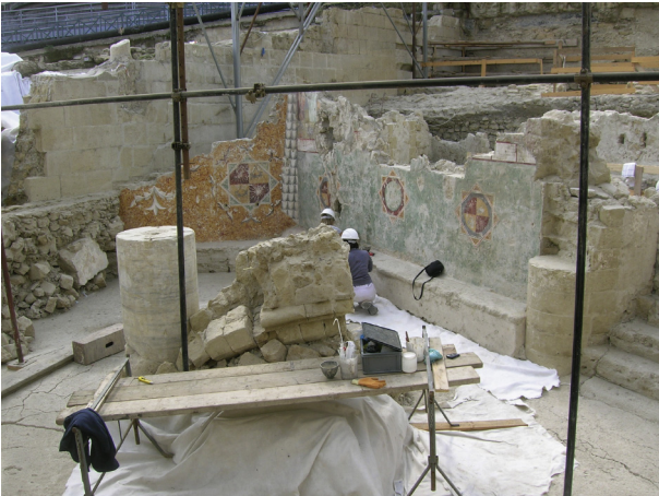
Fig. 8. Municipio Station displays an excavation of the Angioino District (XIII century). (Source: Archives of Metropolitana di Napoli S.p.A.)
