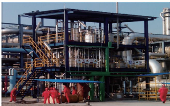
Figure 5. The pilot device at Puguang for the mineralization of flue-gas CO 2 using PG.
