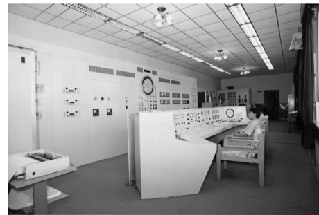
Fig. 7 Main control room of HWRR-II
