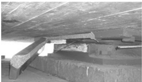
图3 盆式支座限位器被破坏 Fig. 3 Failure of restrainer
