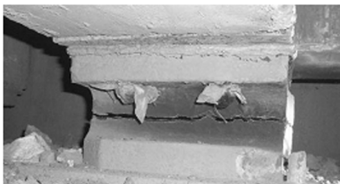
图4 固定支座被剪坏 Fig. 4 Fixed bearings are sheared
