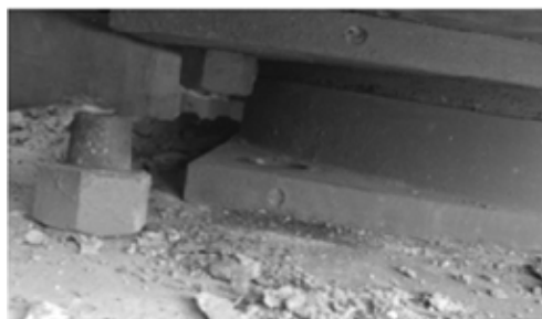
Fig. 1 Bolts are sheared
